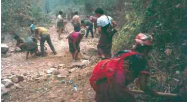
Villagers are forced to build a road as part of the SPDC's border area development program.
