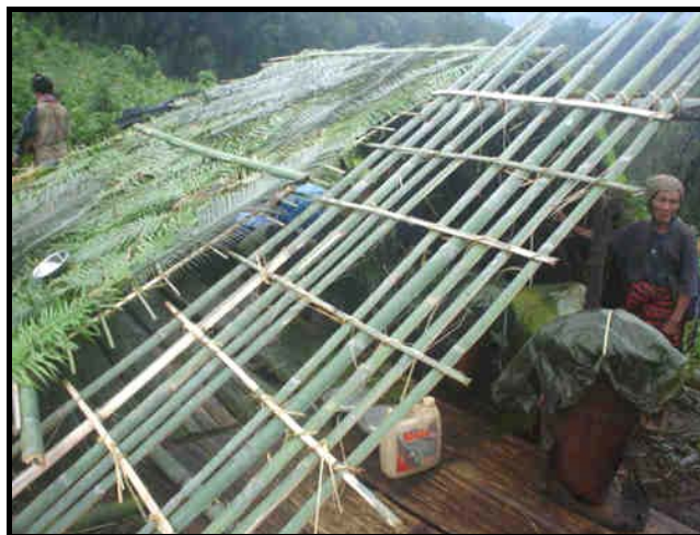
Karen IDPs constructing shelters in the forest in the Yeh Mu Plaw area, Papun District in June 2006. [Photo: FBR]
